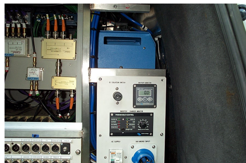
Phoenix MultiPlus and associated control gear installed on Sky News satellite News gathering vehicle.
