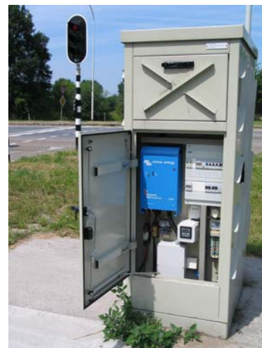
Installed backup power installation
