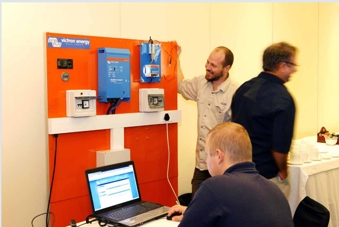
Photo 2: VGR software can be used to remotely configure a system.
