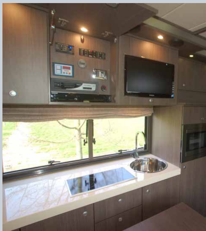
Photo 1: The BMV and the Digital MultiControl Panel from Victron Energy, installed in the horsetruck.
