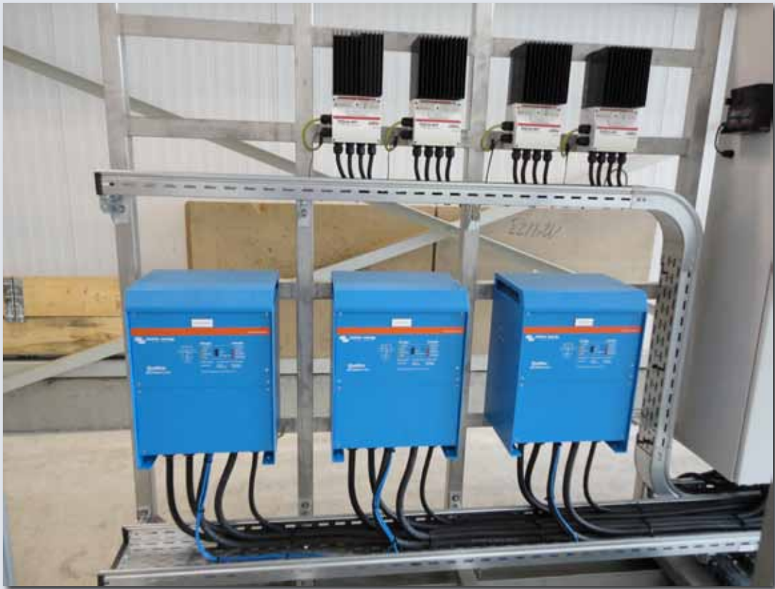
Photo 1: Three Victron Quatro's at the center of the solar energy system.
