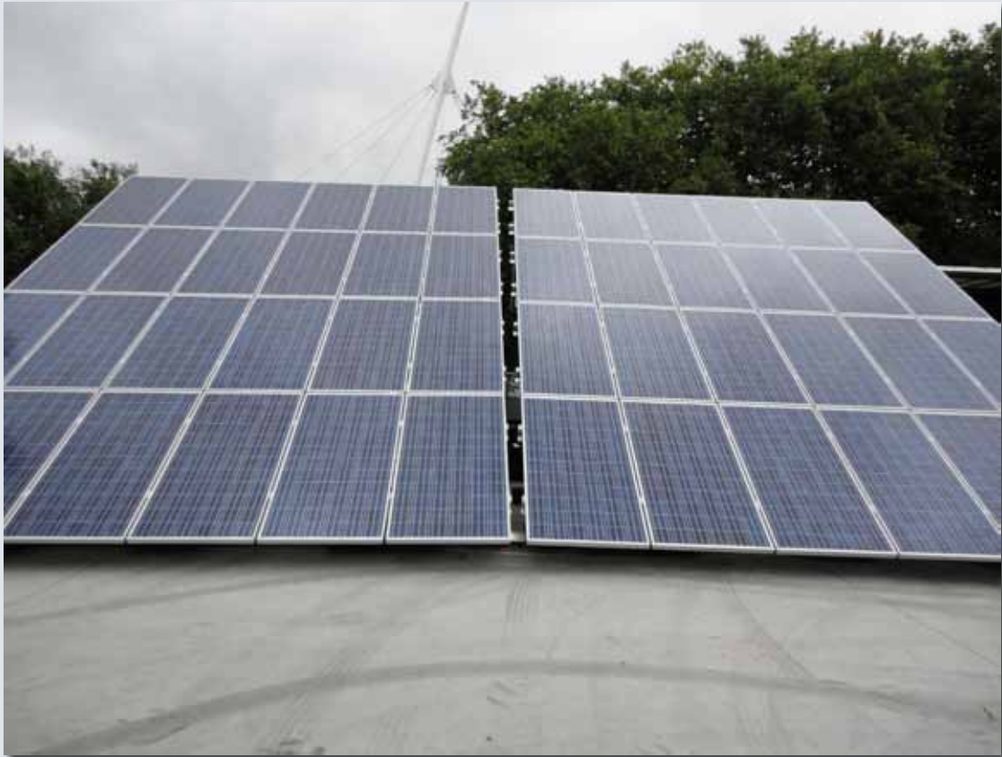
Photo 3: 40 solar panels at the roof of the REN-Mobile.
