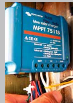
The Victron 75/15 installed alongside my battery box
