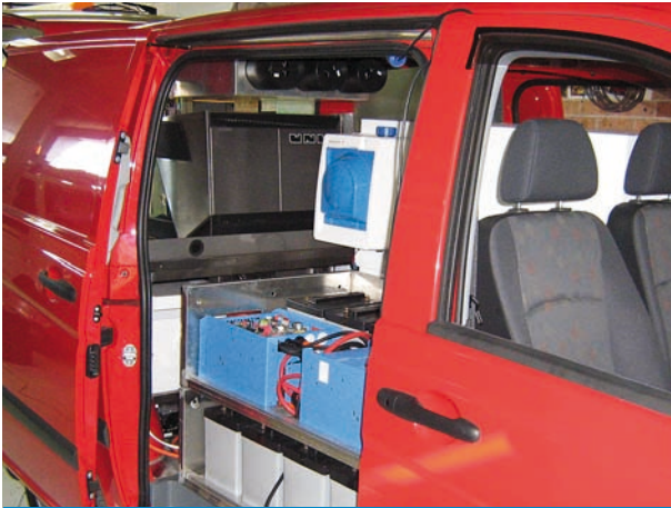
Installation of two paralleled Victron Energy MultiPlus 24/3000 inverter/charger units and battery bank.
