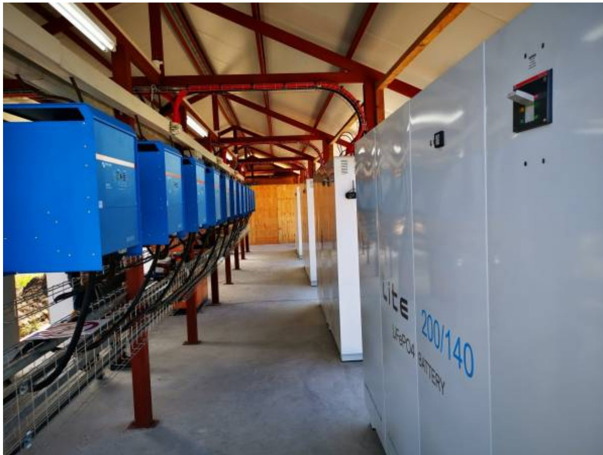
Figure 2 Typical Installation: 7 x Freedom Won LiTE Commercial 200/140 with Victron 12 x 15kVA Quattro and 10 x Ve Direct MPPT's and 6 x Fronius ECO 27kW
