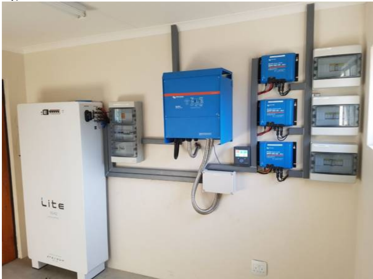
Figure 1 Typical Installation: Freedom Won LiTE 60/42 with Victron 15kVA Quattro and 3x Ve Direct
