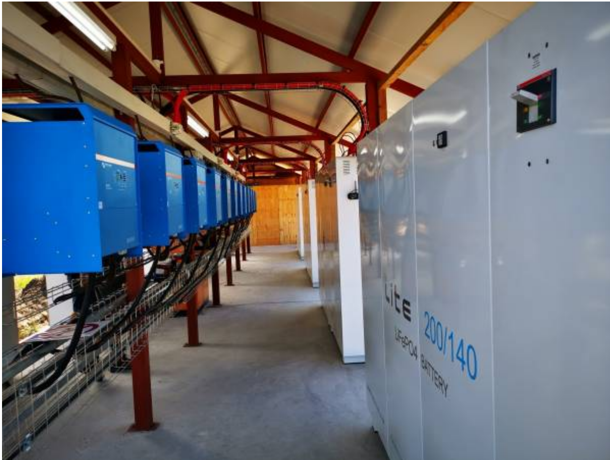
Figure 2 Typical Installation: 7 x Freedom Won LiTE Commercial 200/140 with Victron 12 x 15kVA Quattro and 10 x Ve Direct MPPT's and 6 x Fronius ECO 27kW
