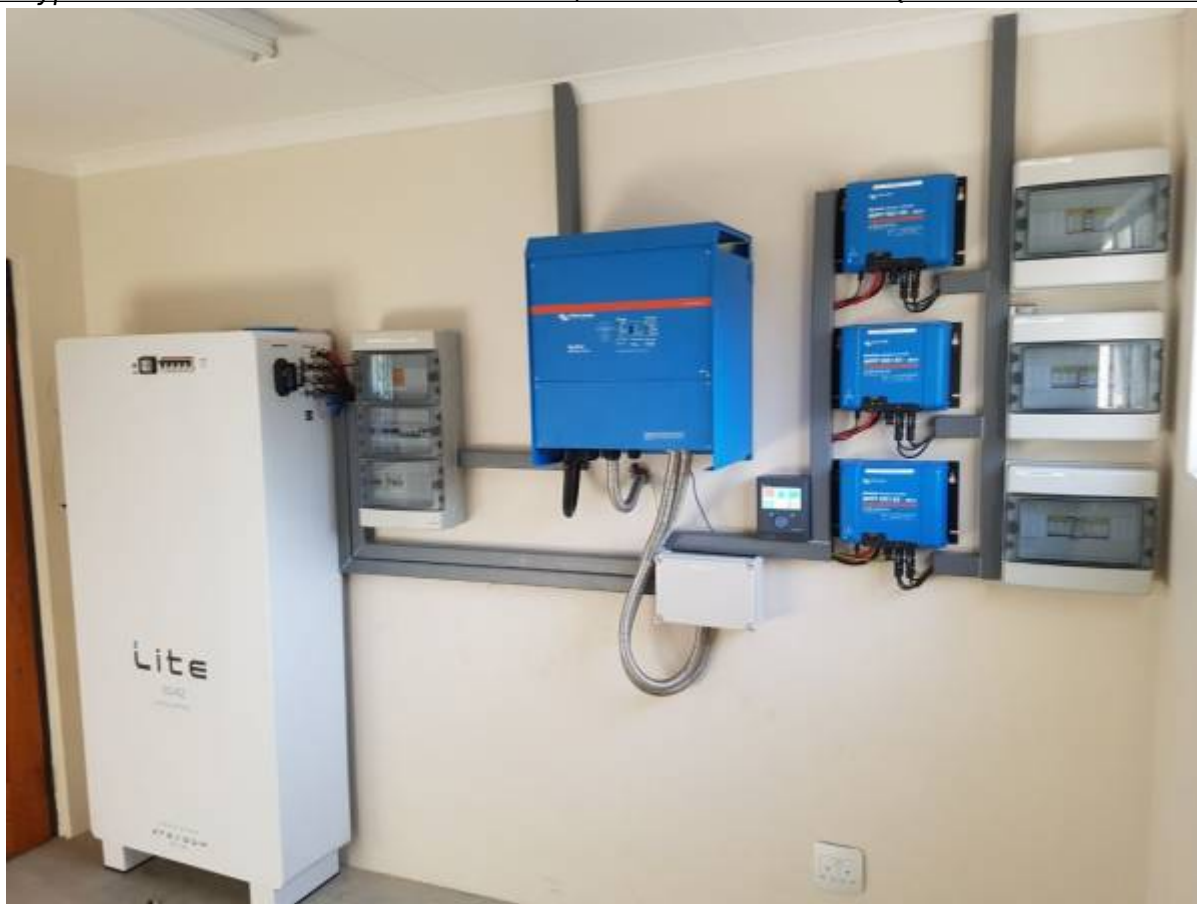
Figure 1 Typical Installation: Freedom Won LiTE 60/42 with Victron 15kVA Quattro and 3x Ve Direct
