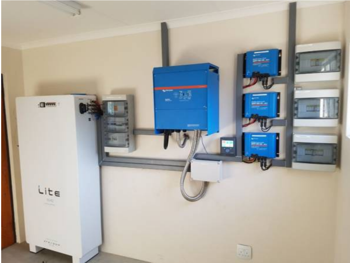
Figure 1 Typical Installation: Freedom Lite 60/42 with Victron 15kVA Quattro and 3x Ve Direct MPPT's
