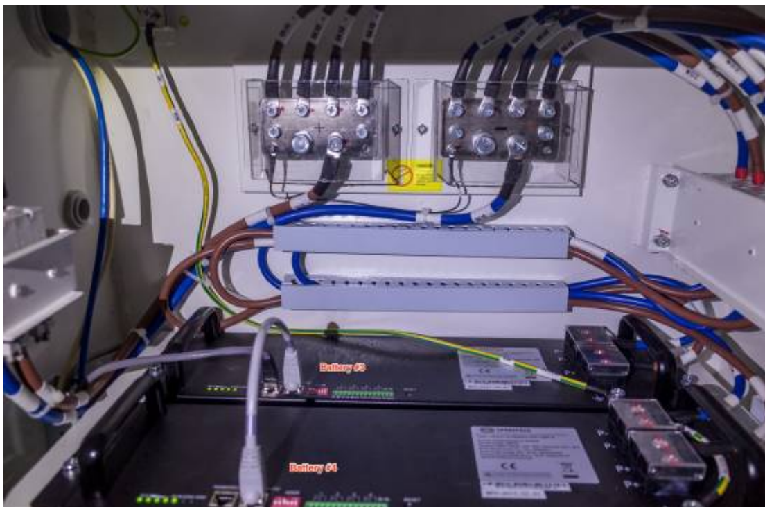
Top two batteries.
