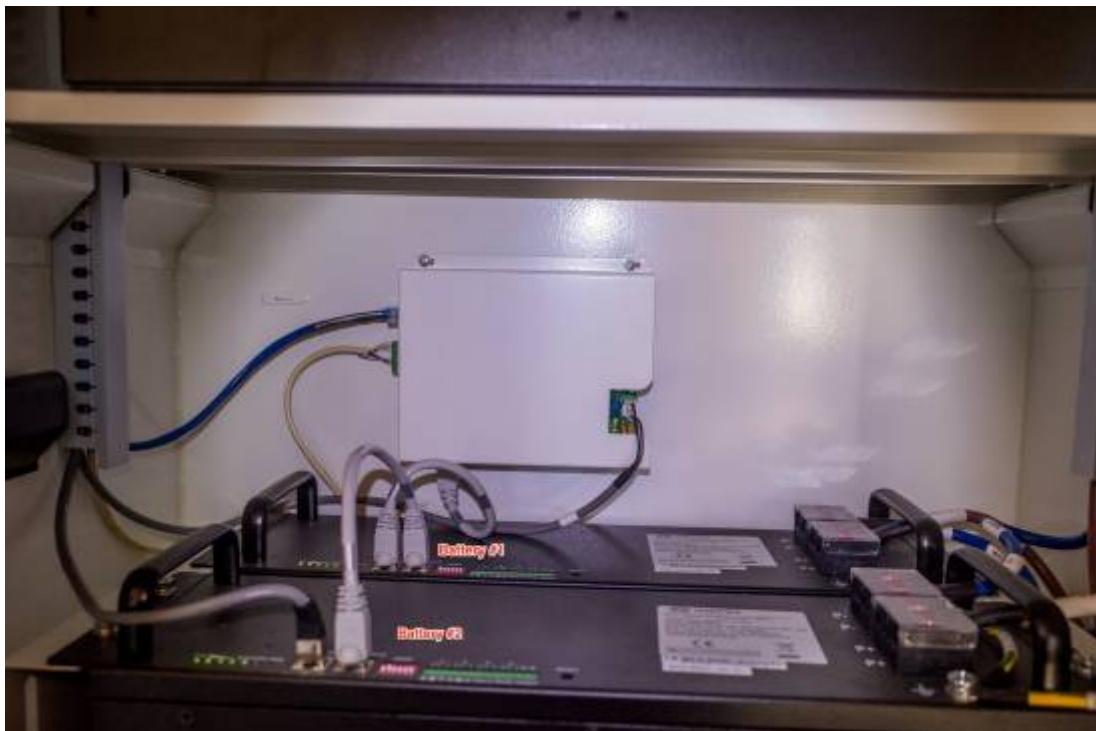
The bottom two batteries.
