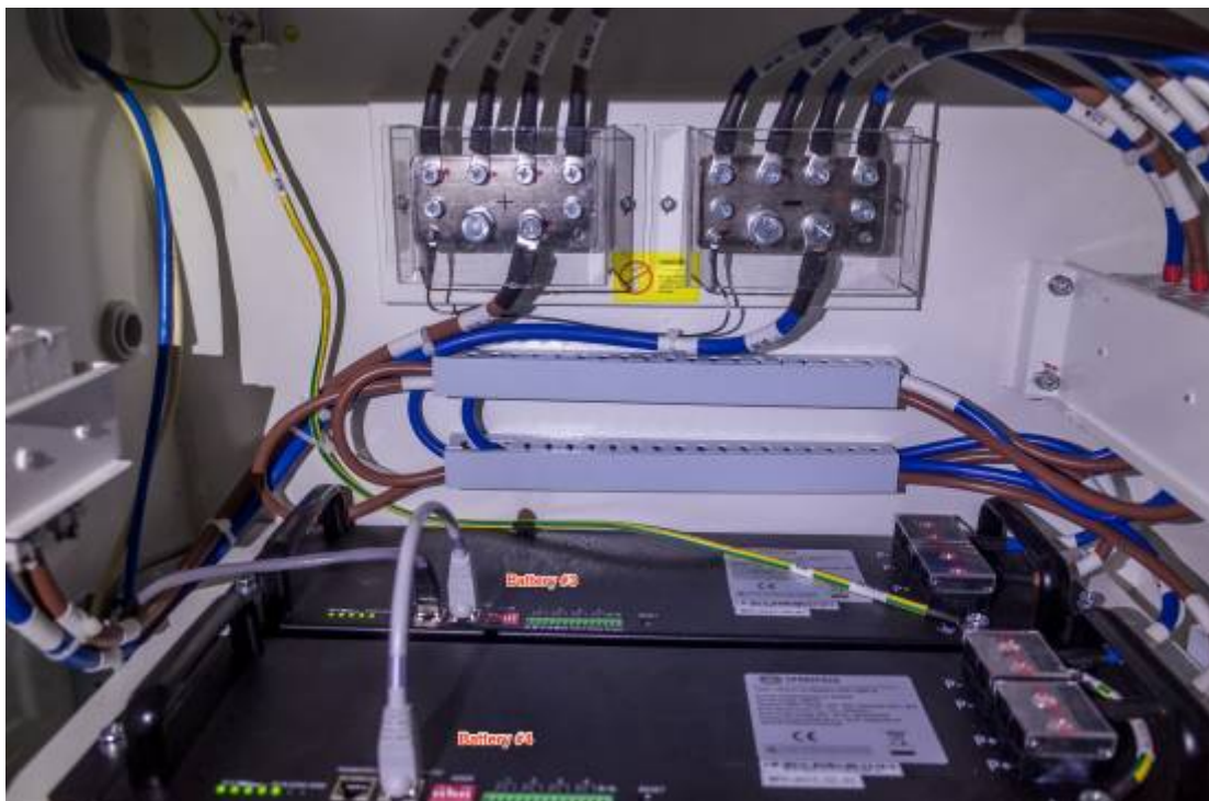
Top two batteries.
