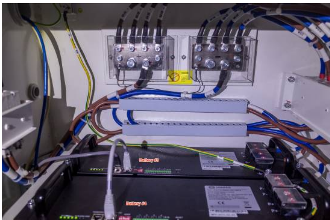
Top two batteries.
