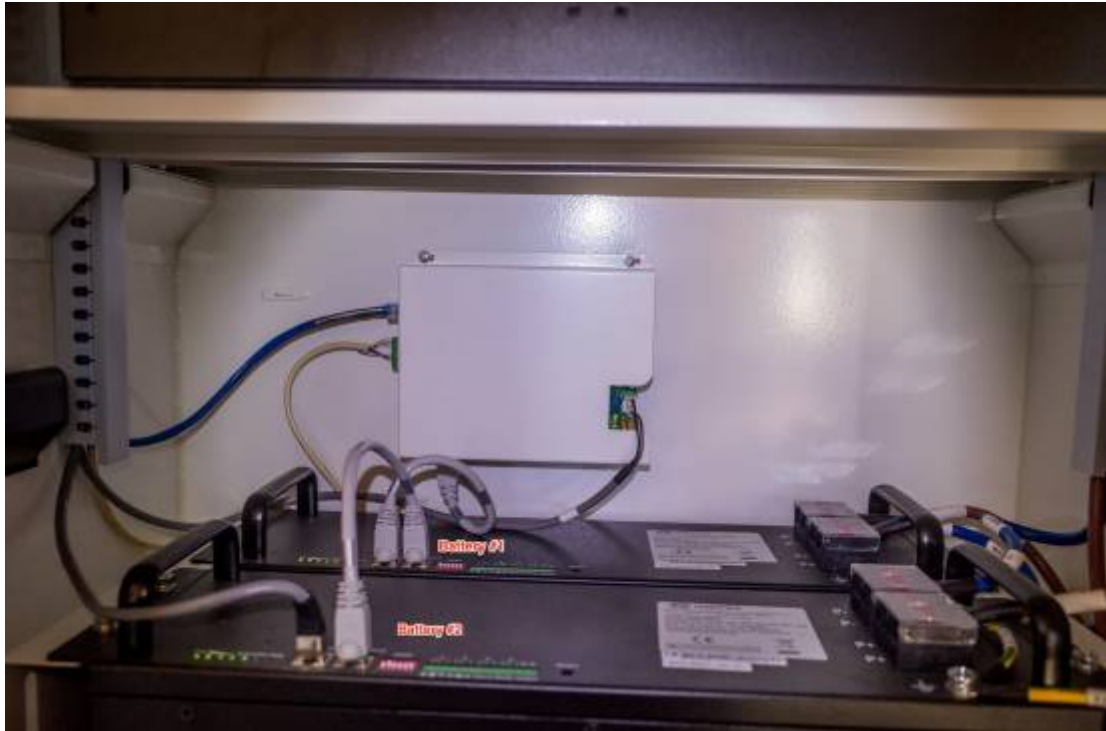
The bottom two batteries.
