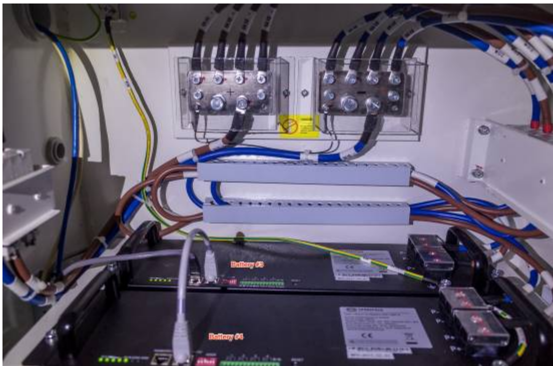
Top two batteries.
