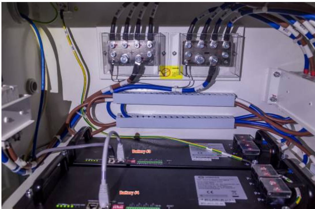
Top two batteries.
