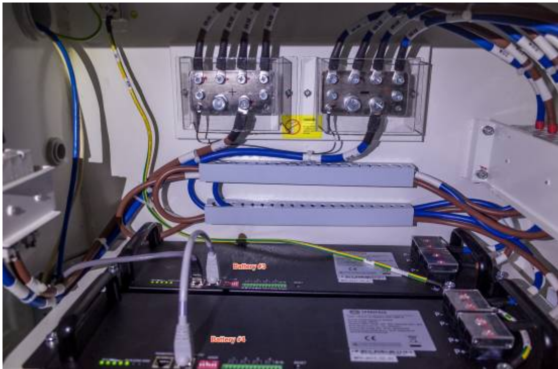
Top two batteries.
