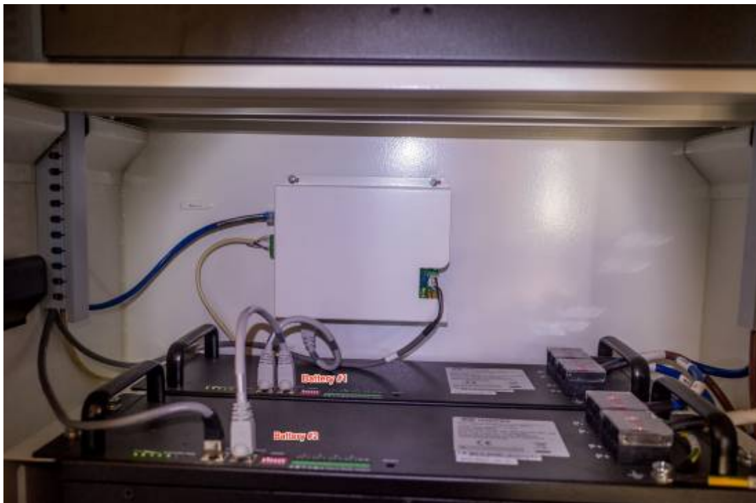
The bottom two batteries.
