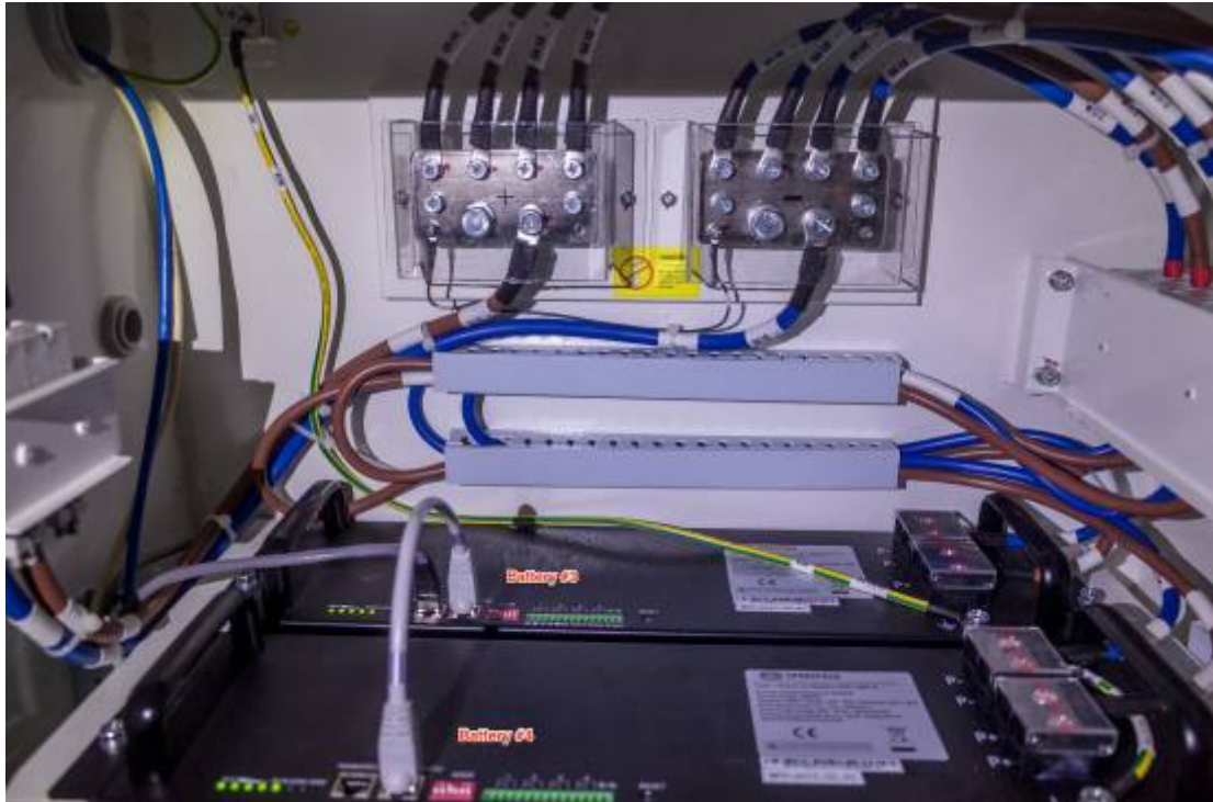
Top two batteries.
