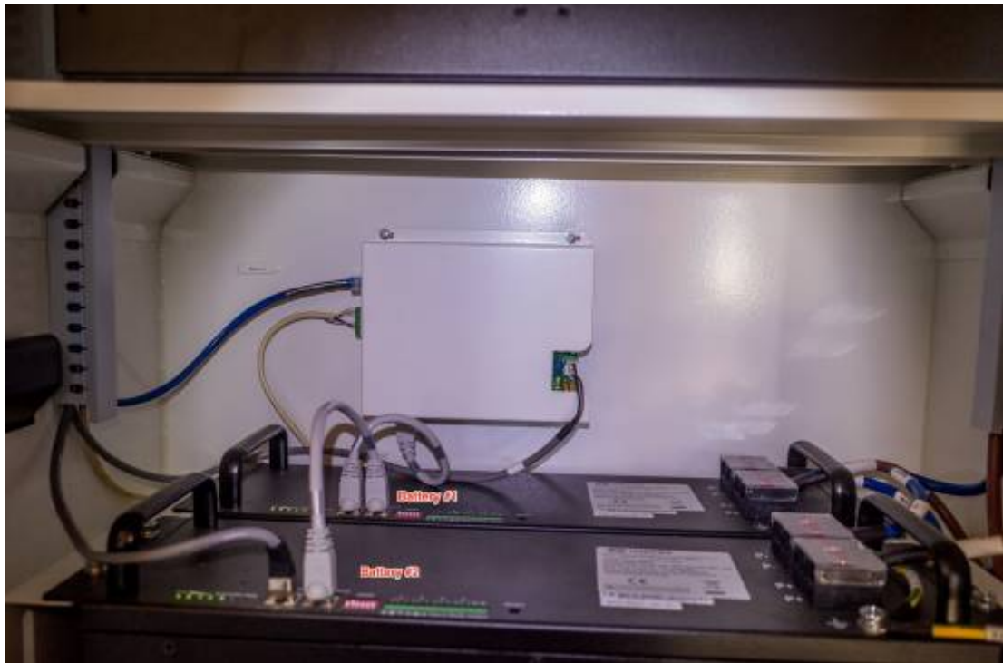
The bottom two batteries.
