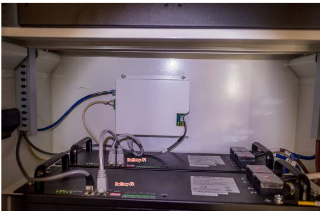
The bottom two batteries.
