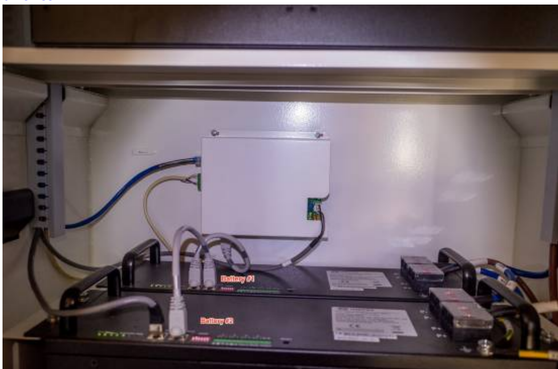
The bottom two batteries.
