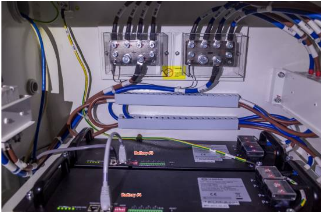
Top two batteries.
