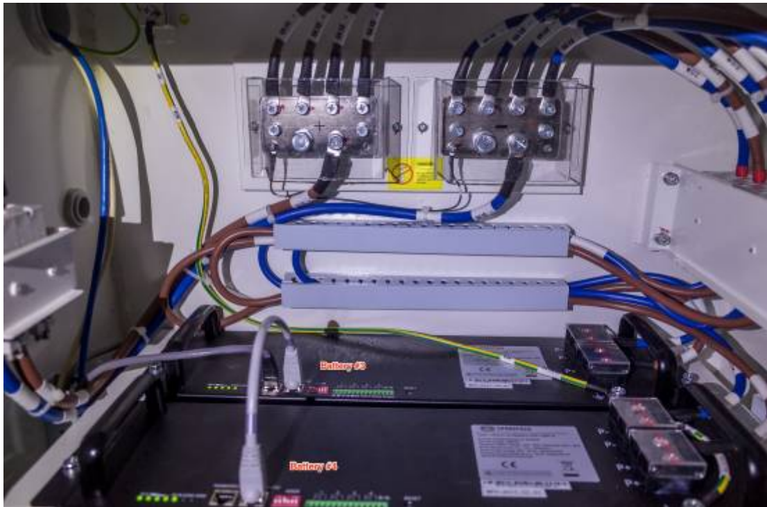
Top two batteries.
