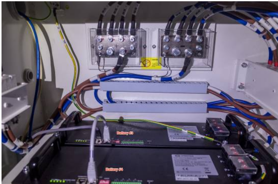
Top two batteries.
