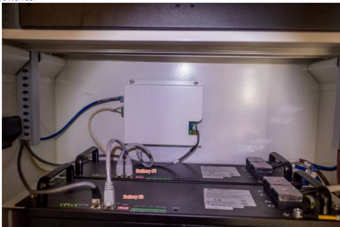
The bottom two batteries.
