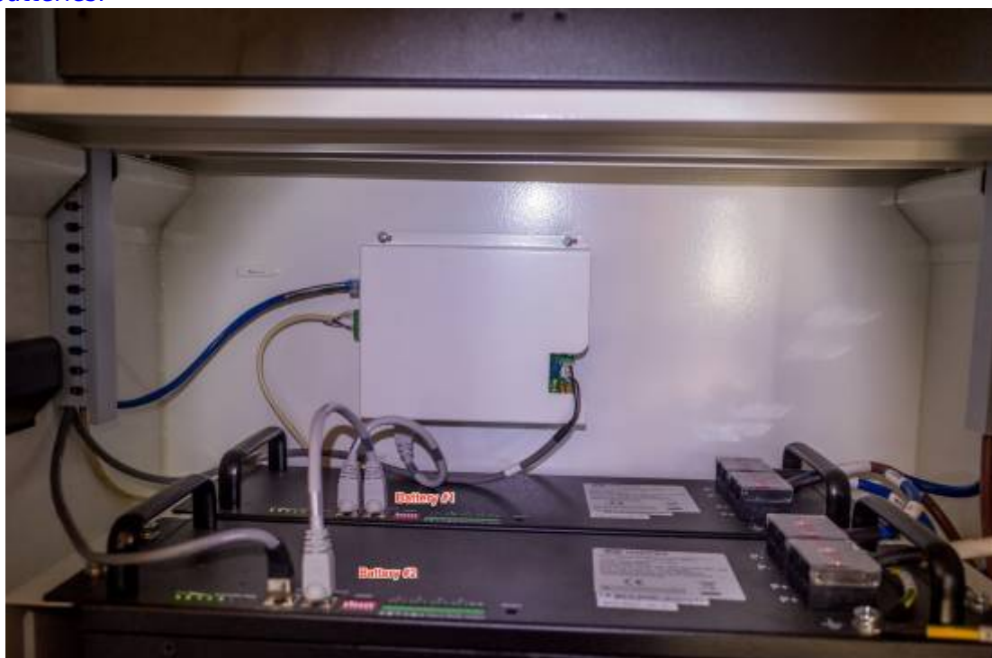
The bottom two batteries.
