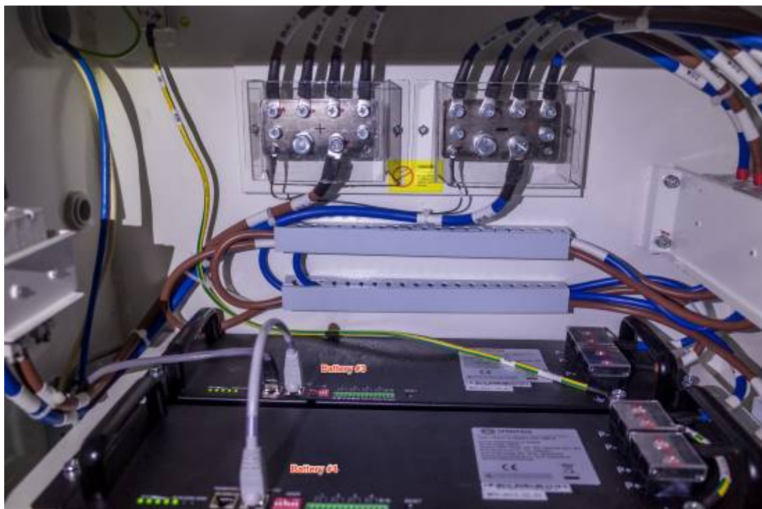
Top two batteries.
