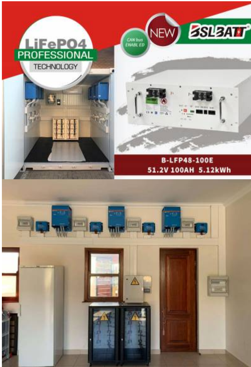
Installation image courtesy of 'Get Off Grid' South Africa.
