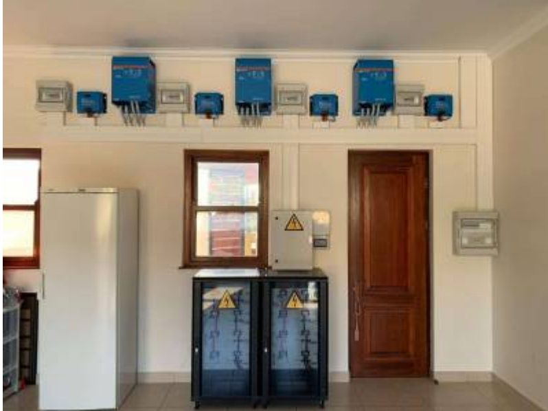
Installation image courtesy of 'Get Off Grid' South Africa.
